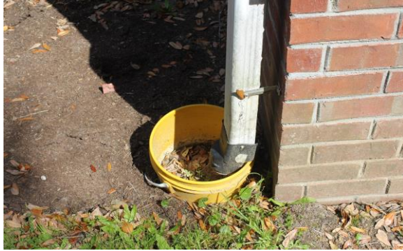
Gutters draining into the side of the house
